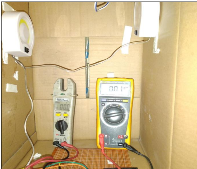
Fig 4.4: Lighting system off due to no presence sensed, hence no measured values being displayed on the digital multi-meters LCDs
