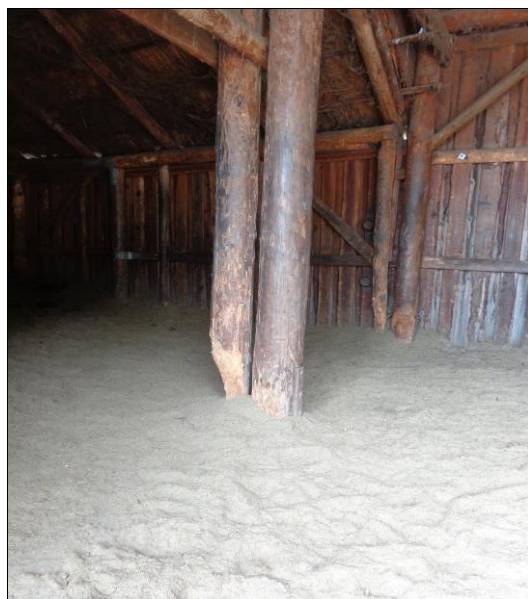
Picture 10: Clearly visible damage to the wooden pillars holding up the canopy roof (Foto: M.Nemecek)
